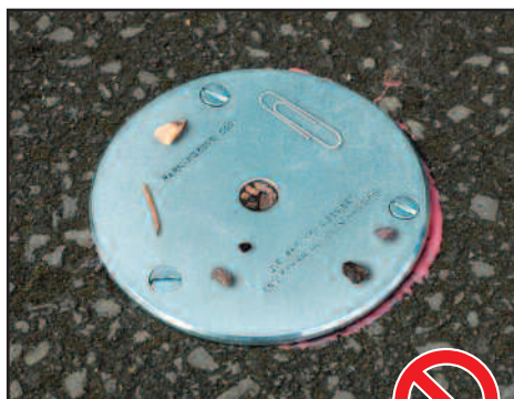
Debris on Base Plate
