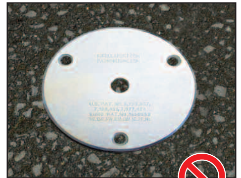
No or Wrong Epoxy
